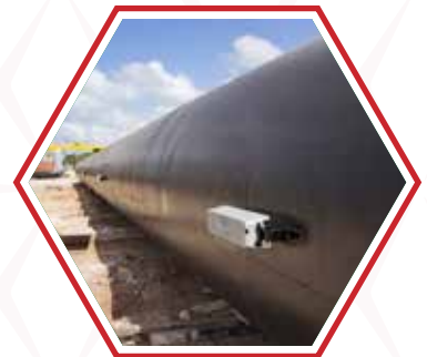
Cathodic Protection Services
